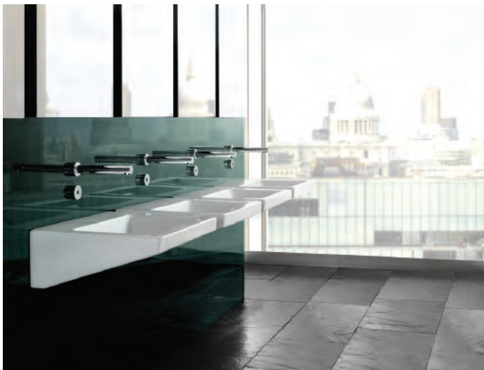
Leadenhall basins with Sensorflow mixers
